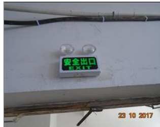
Photo of the inside of the main production hall Exit sign and emergency light.JPG
