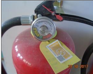
Photo of fire safety equipment Functional fire extinguisher.JPG
